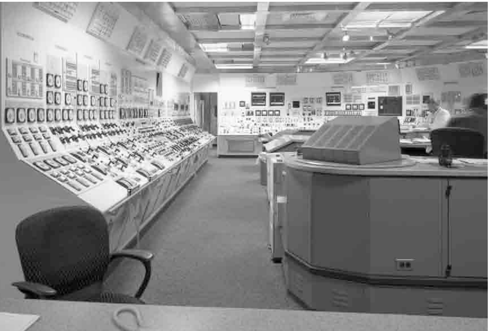
Unit 1 Control Room.
